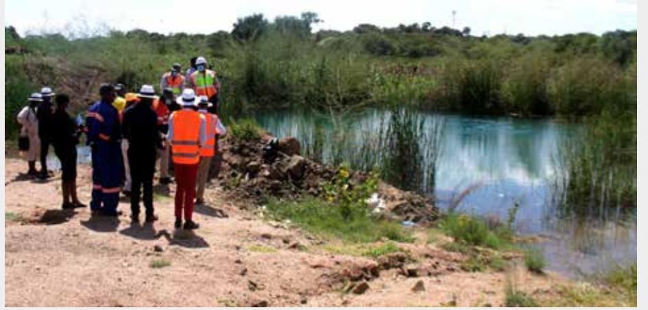
Water Utilities Corporation (WUC) briefed the media on the planned shut down Oodi-Mmamashia North South Carrier pipeline to fix a major leak on the pipeline. The shutdown will start from 24 March until 26 March 2022, resulting in water supply interruption in Mochudi, Lobatse, Gaborone and surrounding areas. WUC chief executive officer Gaselemogwe Senai briefed the Media at site where the fixing will take place. (Pic:PRESS PHOTO)
